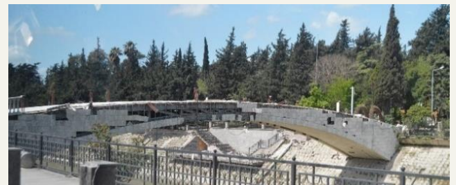
Fig. 7 Pedestrian truss bridge with non-structural damage, Antakya
