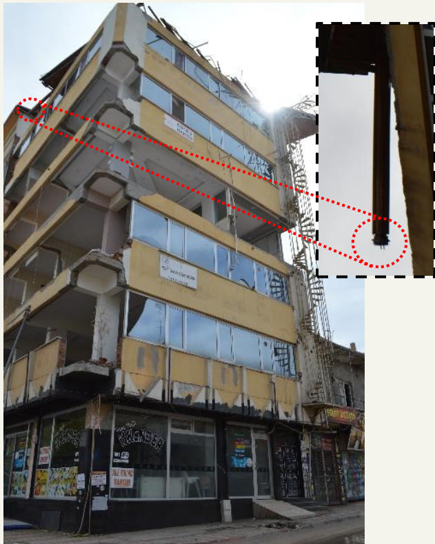
Fig. 5 Total collapse of top floor steel roof due to insufficient anchorage and bracing, Pazarcık
