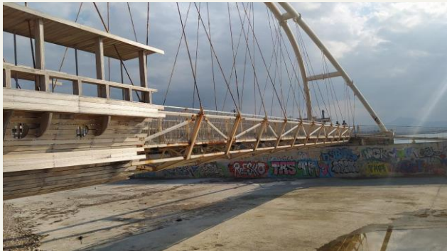
Fig. 3c Structural assessment of an existing arch pedestrian bridge in Corinth [48.50 m] (Konstantinos Fasoulakis, 2024)
